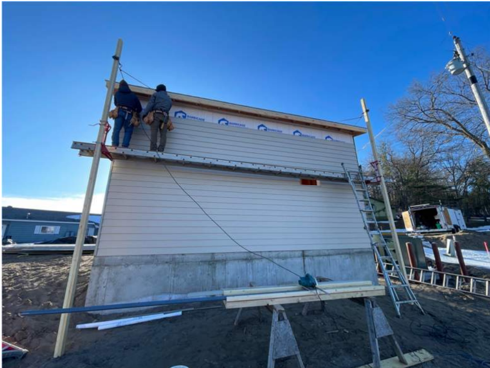
Photo #4: Continuing to install metal siding along the back side of the pump house - Apr 3, 2024, 8:38 AM
