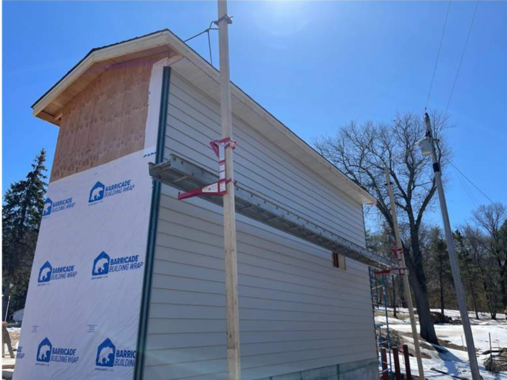
Photo #7: White soffit installed on the back side of the pump house - Apr 3, 2024, 1:03 PM
