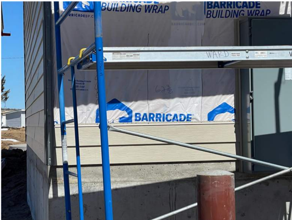
Photo #8: Starting siding along the South side of the pump house - Apr 3, 2024, 1:35 PM
