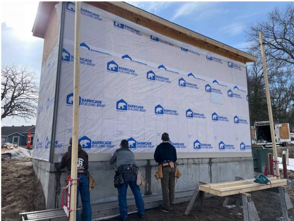
Photo #2: Beginning to nail down the metal siding on the back side of the pump house - Apr 2, 2024, 9:54 AM
