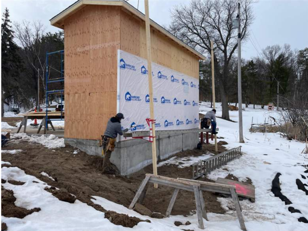
Photo #1: Wrapping the outer walls of the building before installing the steel sheeting - Apr 1, 2024, 10:45 AM
